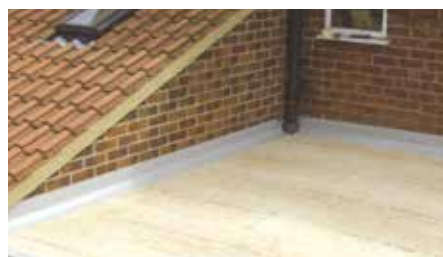
Any other protrusions such as pipes, skylights or other potential weakspots should also be laminated around/over at this point. Any joints between trim lengths are bandaged over.
