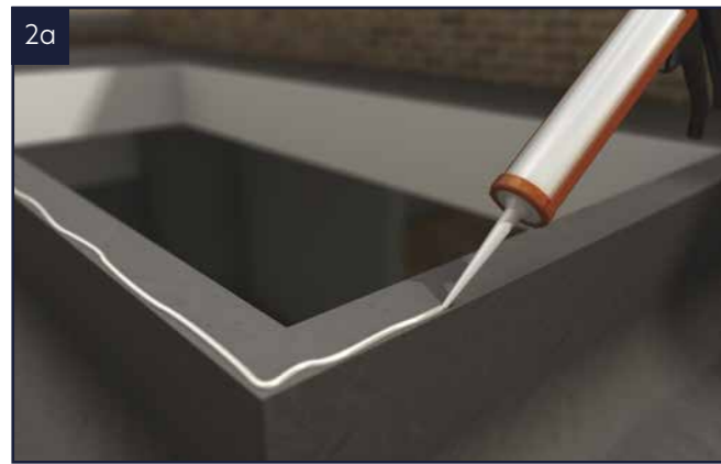
2a Apply a continuous bead of sealant to the outer edge of the upstand.
